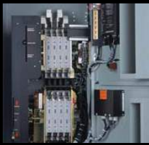
Automatic Transfer Switch
