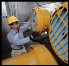
Air System Service
